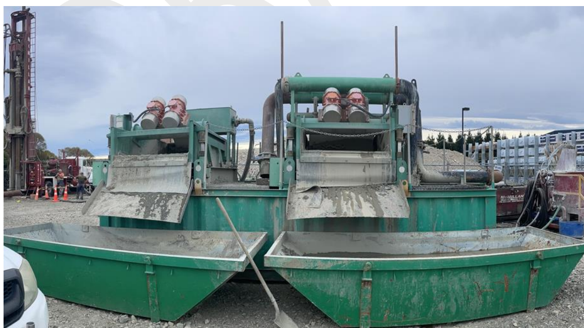
Figure 2 – Solids control units
