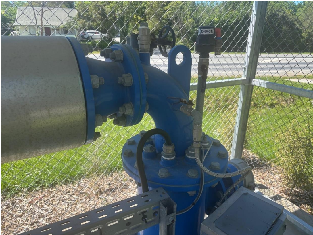
Figure 17 – Drinking water supply bore head componentry
