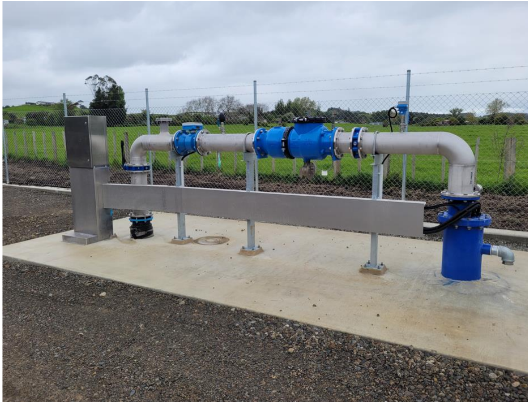
Figure 15 – Drinking water supply bore head
