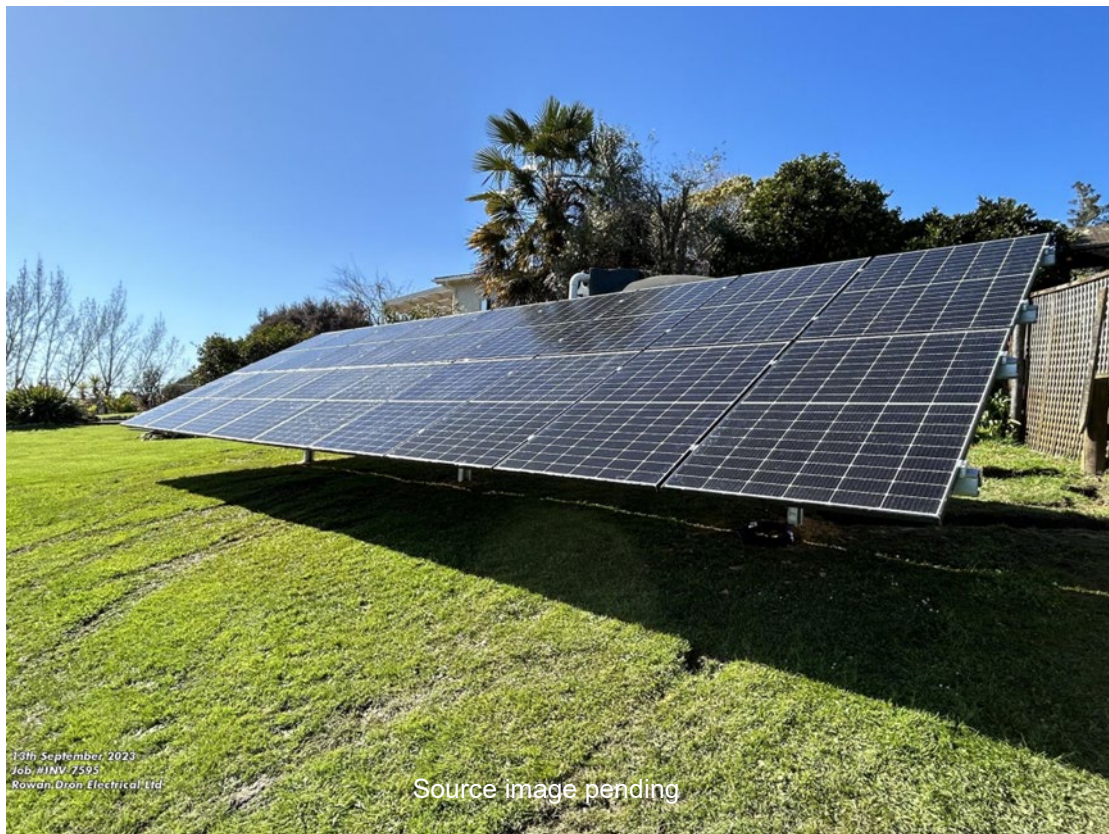
Figure 17 – Example ground mount solar array
