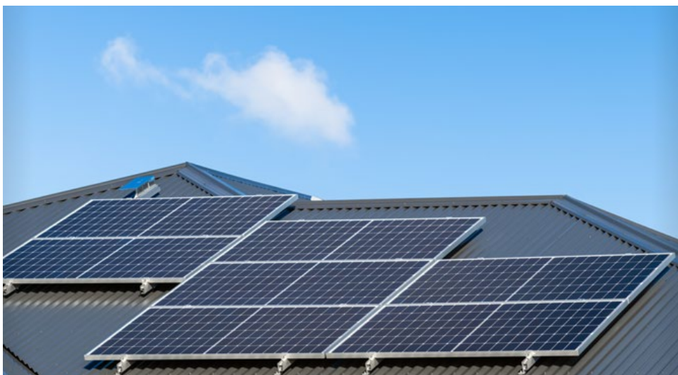
Figure 6 – Typical rooftop solar panel system
