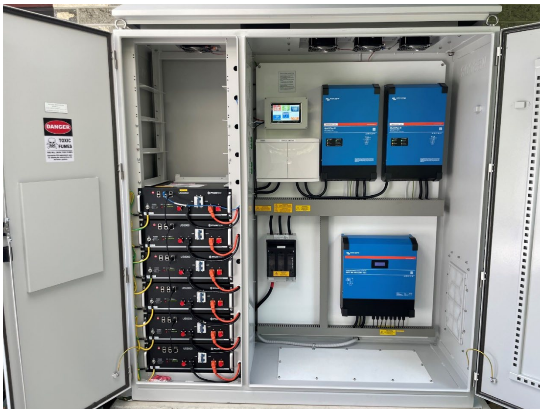
Figure 22 – Typical PCE arrangement
