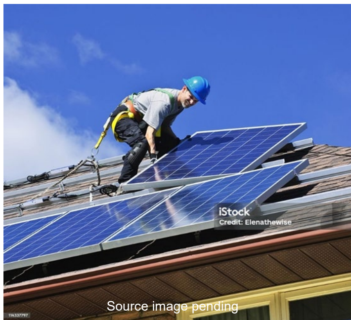
Figure 1 – Typical rooftop solar panels
