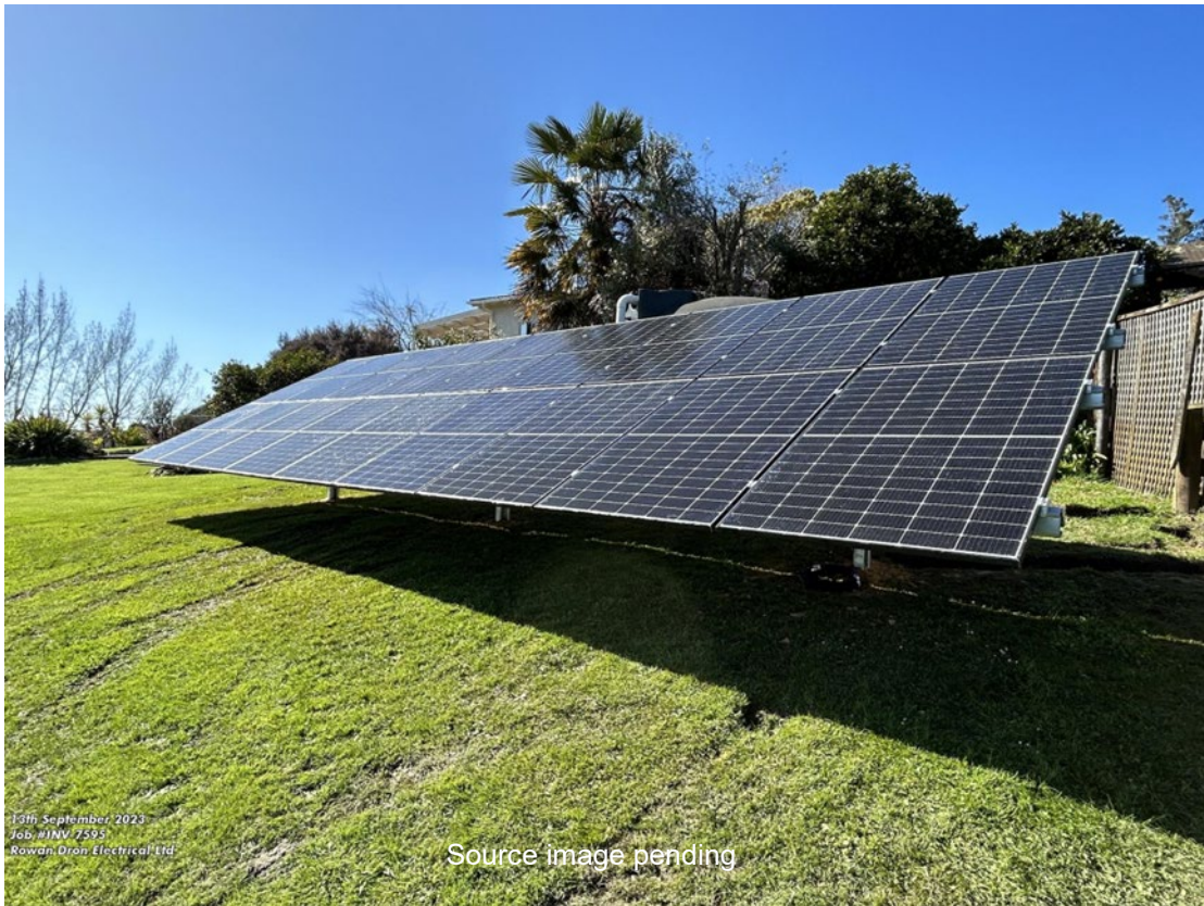
Figure 17 – Example ground mount solar array
