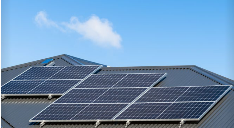
Figure 6 – Typical rooftop solar panel system
